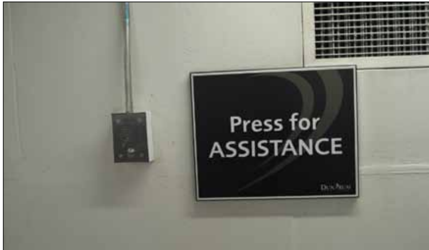
Image 1.20 Example of assistance via an intercom system for car park users.
