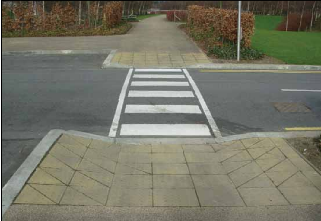
Image 1.35 Example of buff blister surface at uncontrolled crossing.
