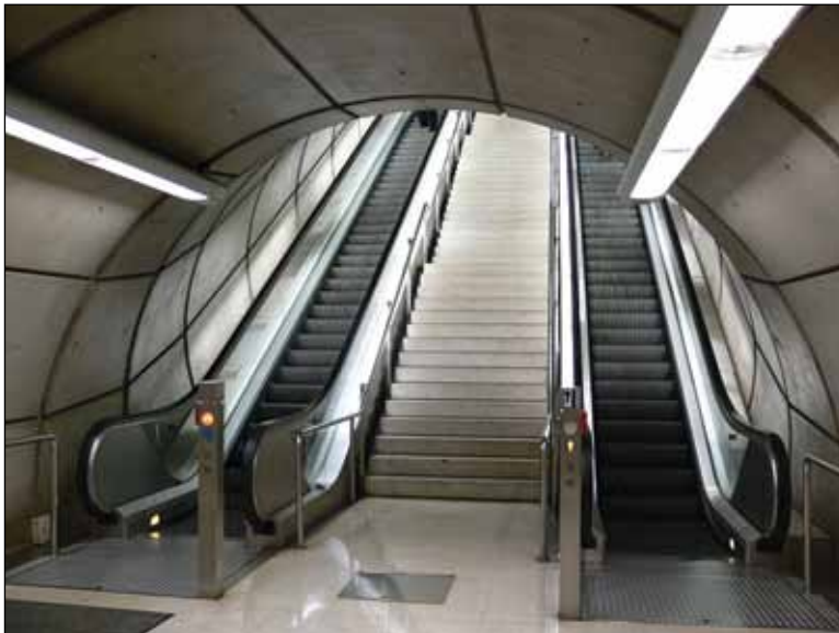
Image 3.20 Example of escalator showing both up and down directions, pole-mounted emergency stop buttons, plus a standard staircase in between.
