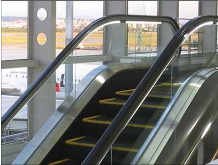
Image 3.19 Example of an escalator with lighting under handrails.
