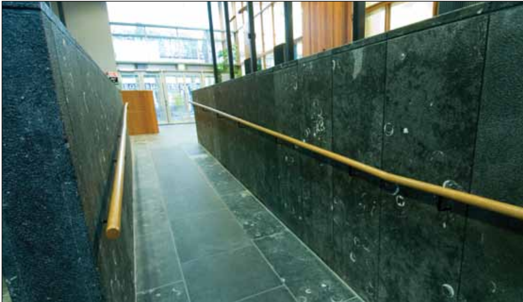
Image 3.3 Example of ramp with selected stone floor surface and contrasting wooden handrails.
