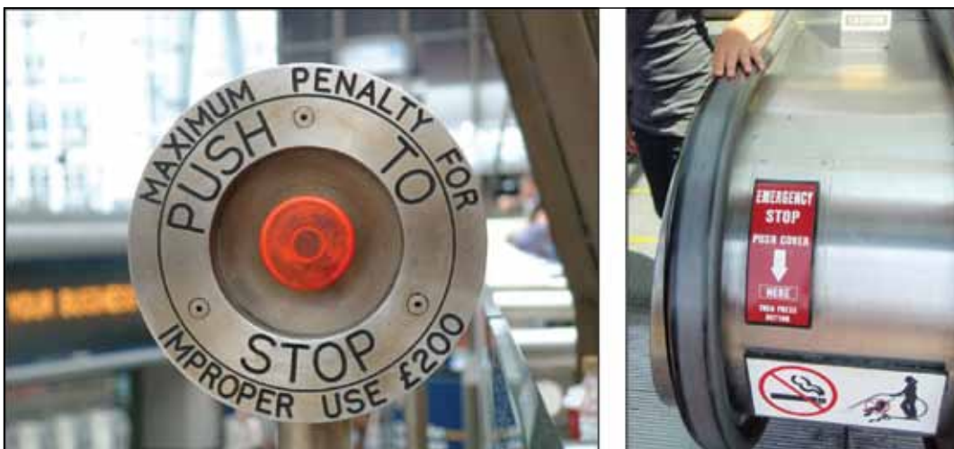
Image 3.21 and 3.22 Examples of escalator emergency stop buttons.
