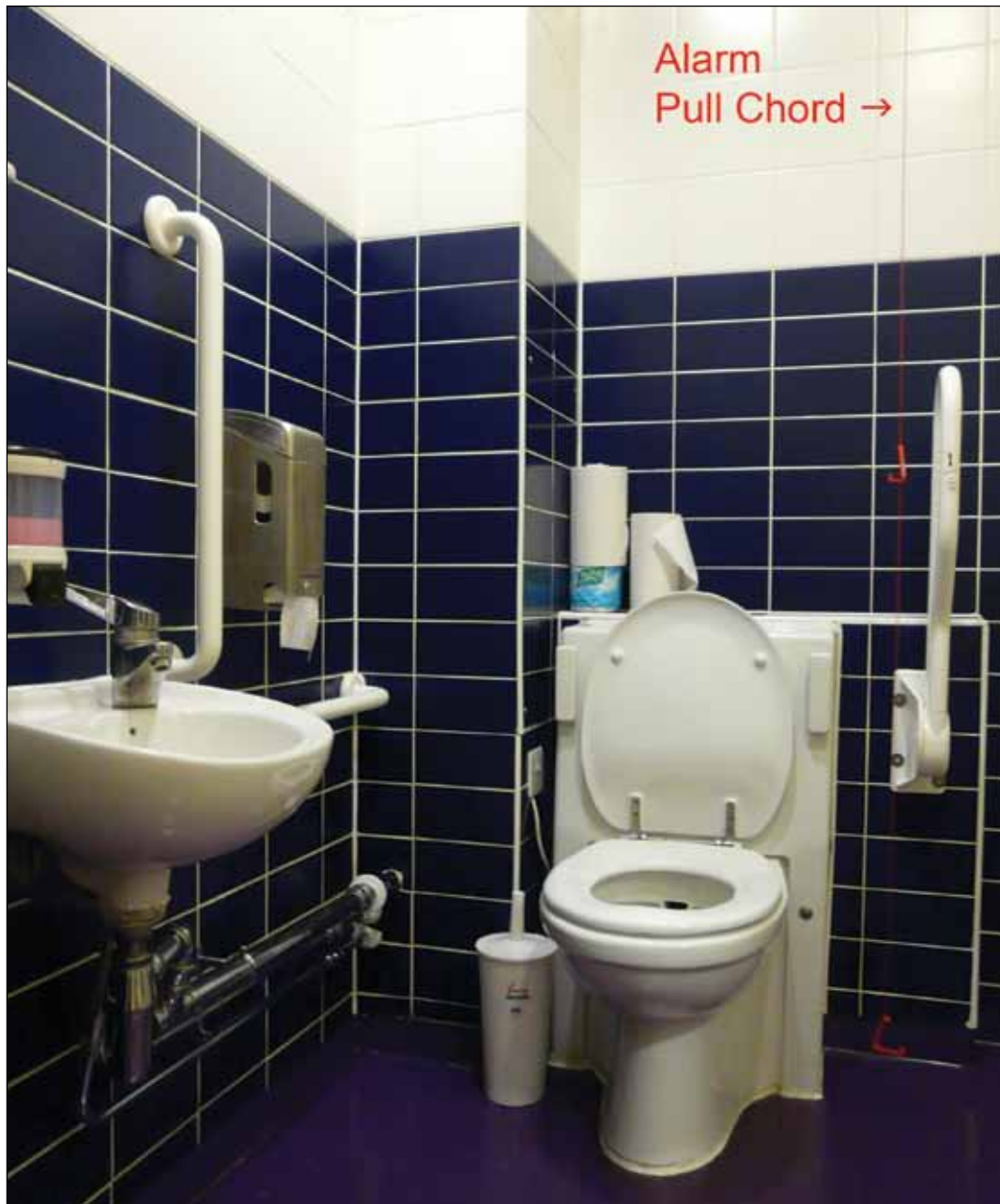
Image 5.22 Example of alarm pull chord with two red bangles in a unisex accessible toilet – Left-handed transfer.
