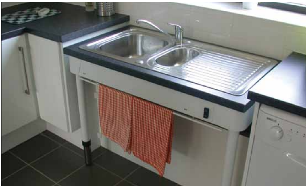
Image 6.12 Example of an adjustable-height, accessible sink. Note the sink may be raised or lowered as suits the user.
