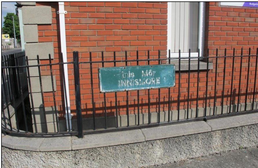
Image 5.1 A poorly maintained street sign.
